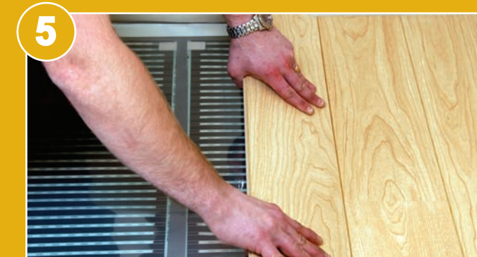
5 Lay the floor covering as soon as possible to prevent damage to the element.
